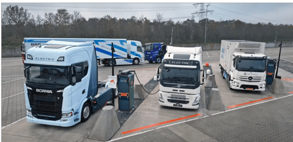
Milence electric truck charging hub, Venlo, Netherlands
